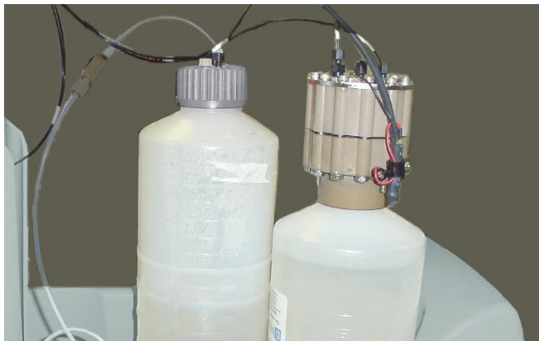
Figure 49. Dionex EGC in the service area
