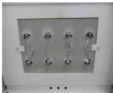
Heating elements connection FAR side
