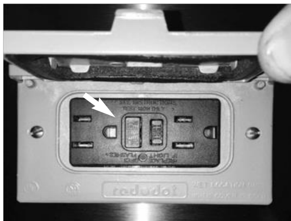
Figure 4-2. Reset Button on GFCI Outlet
