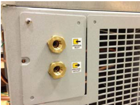
Figure 3. Water line connections on the freezer
