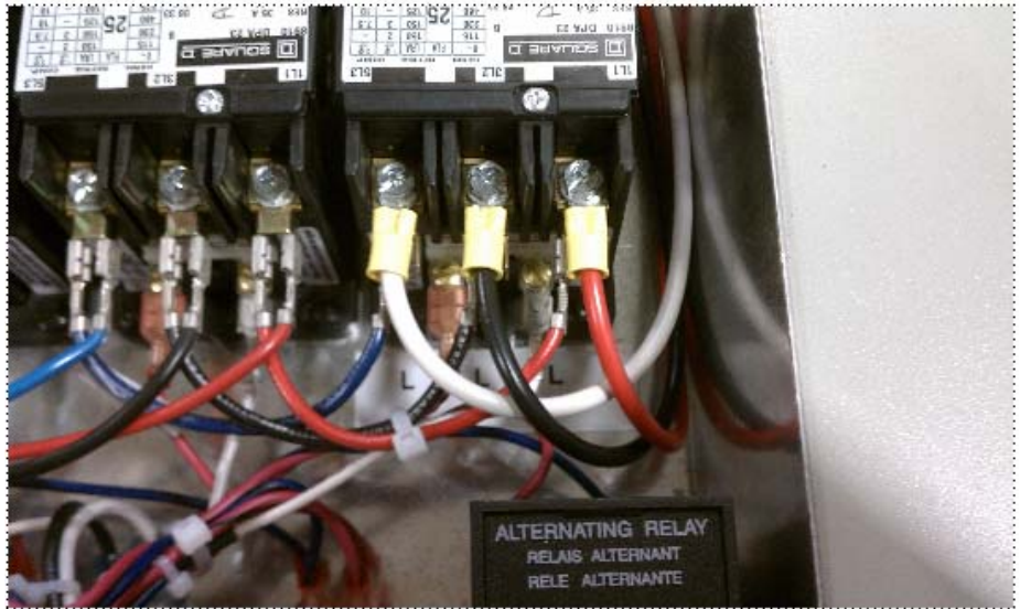
Figure 3. Incoming Power Wiring
