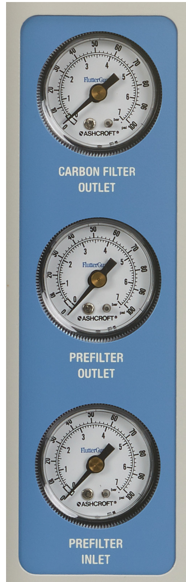
Figure 11. Pretreatment system gauge
