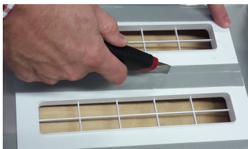
Figure 49. Cut sealing tape between pre-filters
